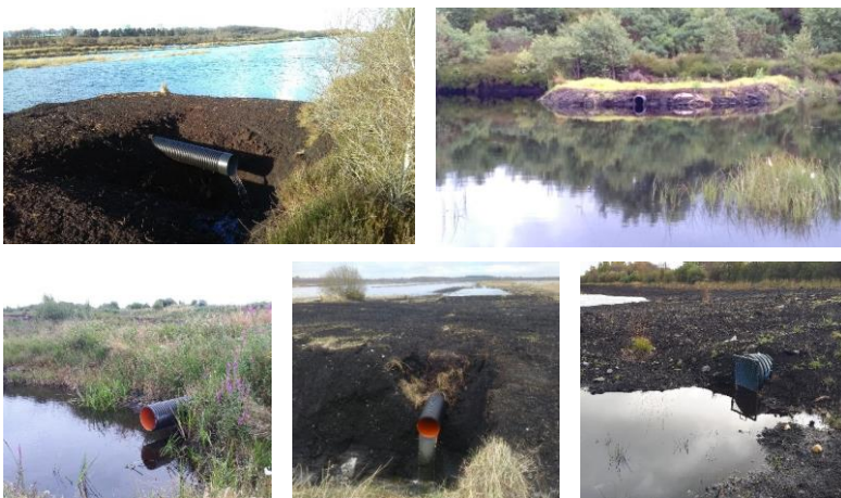
Figure 6: Examples of installed overflow pipes
