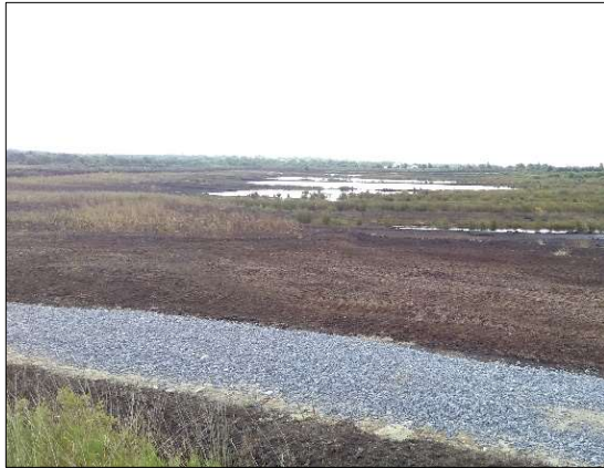
Bare peat along the headlands with the new track at the north-east basin.
