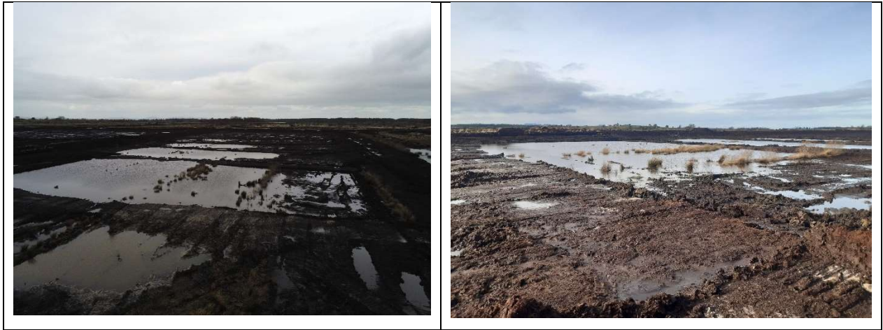
Figure B2.2. Killeens Trial Area Fields levelled with a dozer creating a series of terraces.
