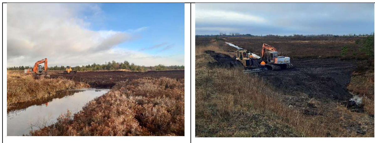
Figure B9.1. Installation of two trench drain blocks at Derryhogan using bulldozer and excavator; note the block on the left photo used mostly peat from surrounding bog; the block on the right used excavated subsoil mixed with peat from the trench drain.
