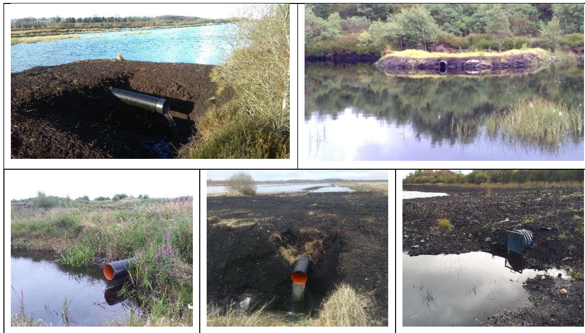
Figure A2.2. The 2 top pictures show the Overflow pipe constructed at Lodge wetland. The bottom left and middle photo is the main water outlet at Cavemount. The bottom right photo is the main water outlet at Corlea. The pipe at Corlea was located at the old pump site.
