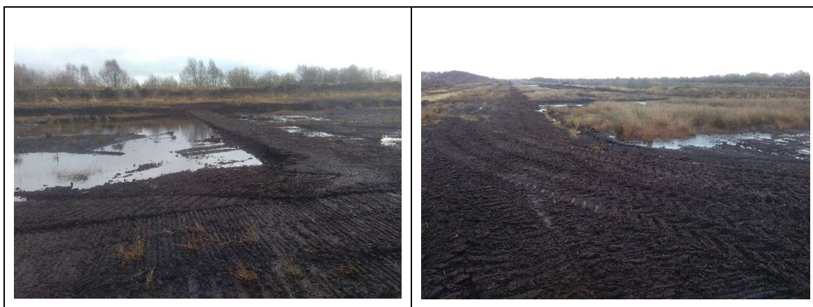
Figure B2.1. Lodge Bog cutaway. Trench bunds were created at Lodge Bog cutaway to create cells to re-wet the cutaway.
