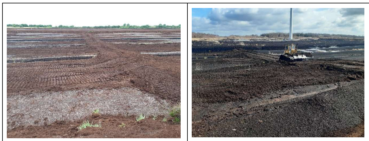
Figure A3-2. Derryvilla Bog (left) and Templetuohy Bog (right): Application of the deep peat cutover bog field drain blocking methodology using a bulldozer.
