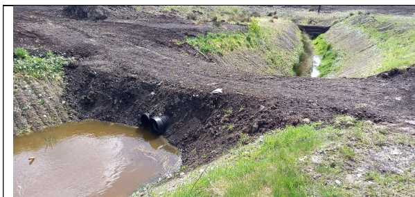
Figure 7.19. Outfall modifications at Mountlucas. The outfall was blocked and a pipe was used to manage water-levels at a higher level.
