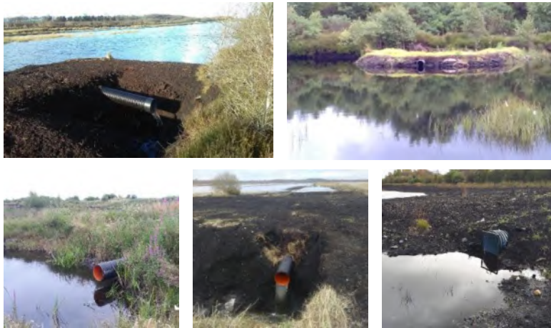
Plate 2-2: Examples of installed overflow pipes
