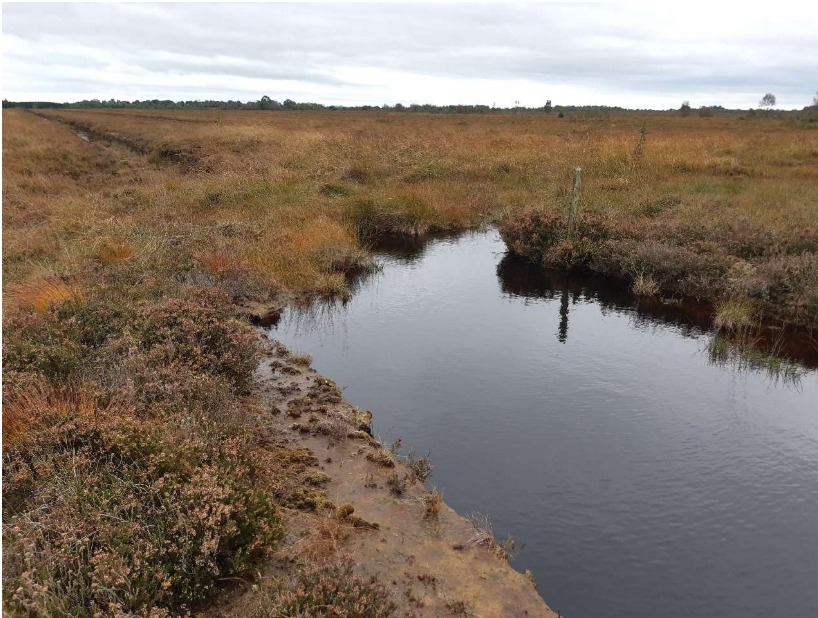
Figure 3.4. View of trench drain blocked by machine pass, water flow has been reduced to a trickle that has overtopped the machine pass at Glenlough.
